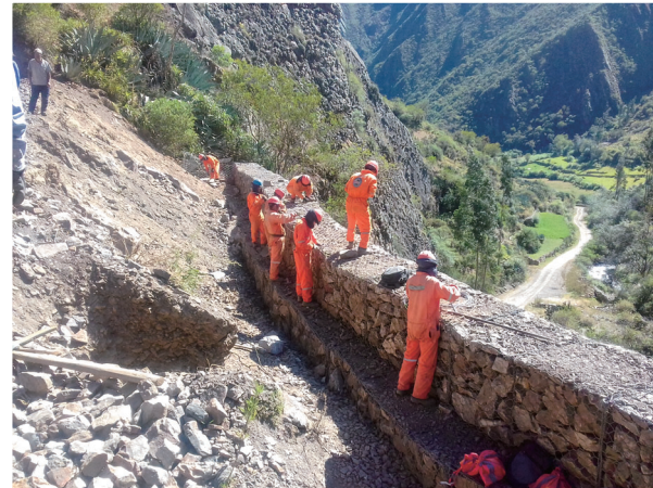
Construction of a debris barrier as a road improvement (Near Llamac Village)
